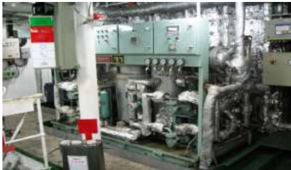
Fuel Units heat, filter and presurmise the treated fuel
