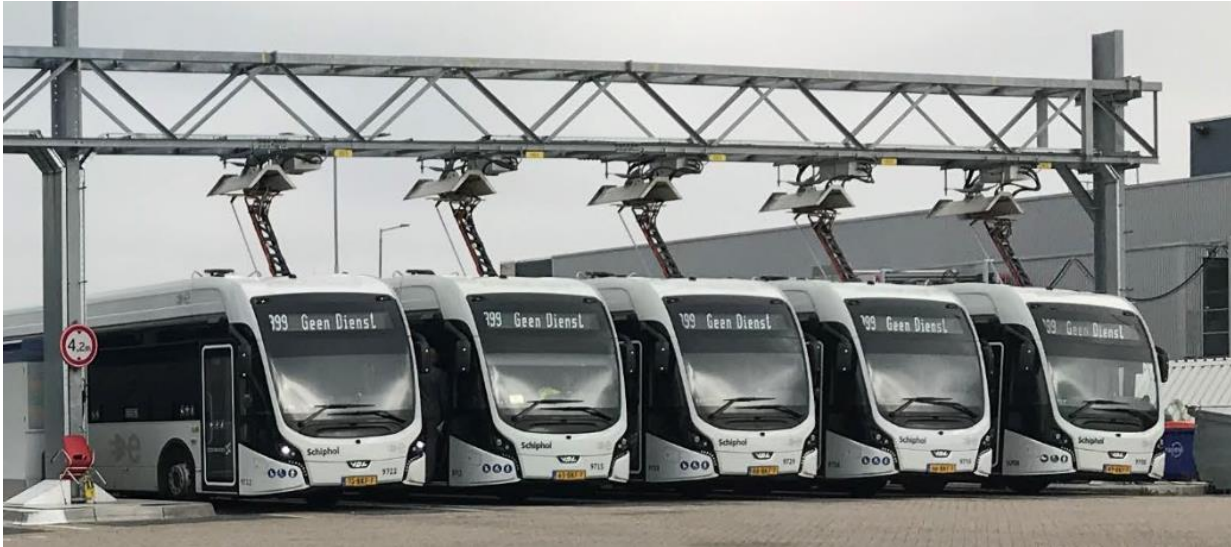
Figure 87 450kW opportunity chargers at the schiphol airport [73]
