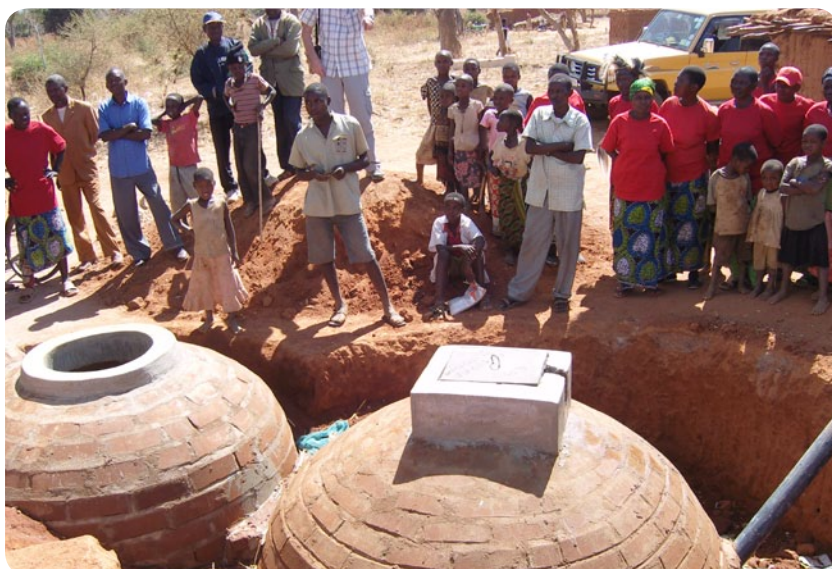
Biogas plant in Tanzania
