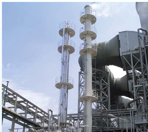
Figure 3.3 Post-combustion capture pilot plant, Beijing (courtesy of Huaneng Group)
