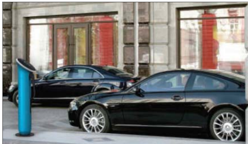
Figure 39 Commercial vehicle charging station
